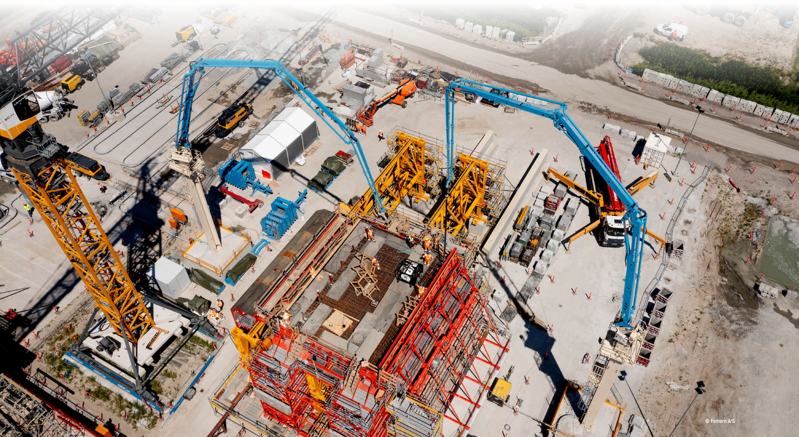
Concreting a tunnel segment with two BSA 2108 HP E stationary concrete pumps and MXR 32-4 placing booms
